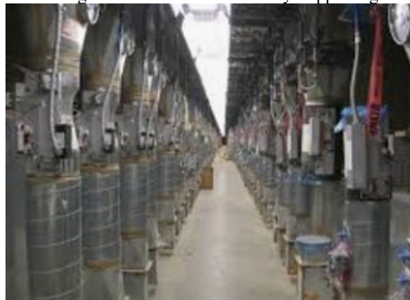
Figure 63 - State-of-the-Art White Oak Infrastructure: Advanced Air Terminal Units Supporting Laboratories
